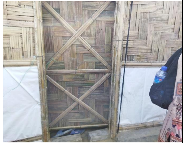
Fence Branding tarpaulin wrong setting
