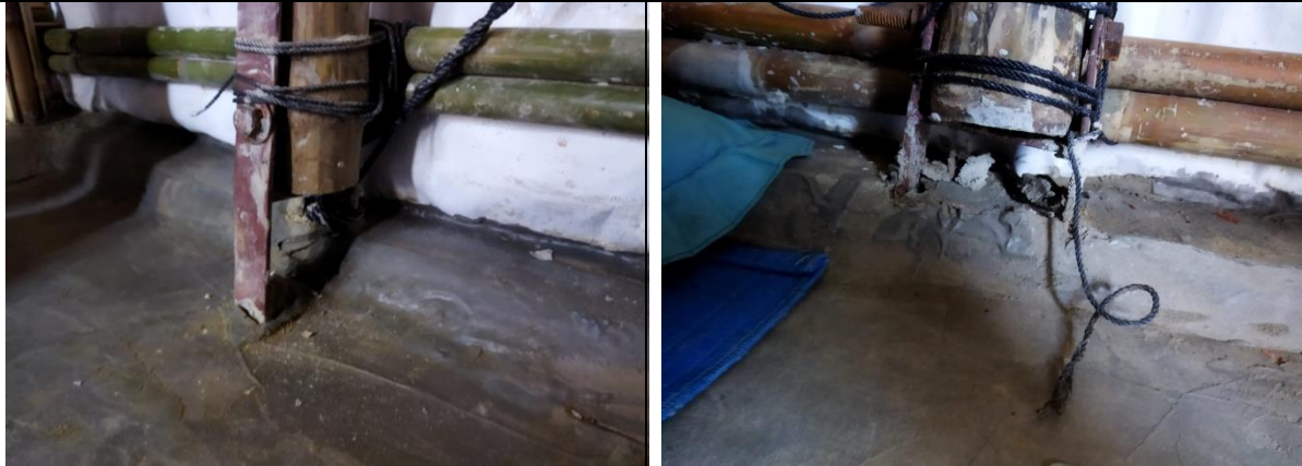
Excess gap between Boark and floor
