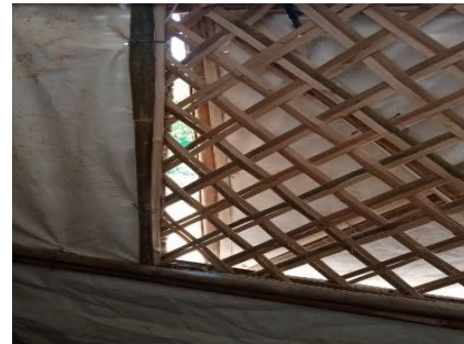
Window wrong setting
