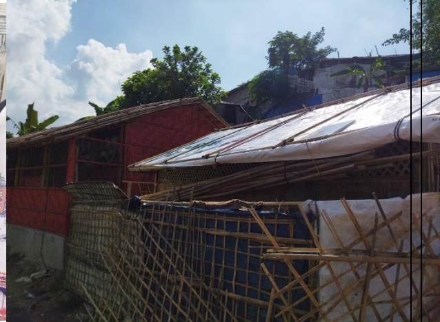
Roof tarpaulin wrong setting
