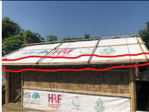
Wrong roof tarpaulin set with Mua
