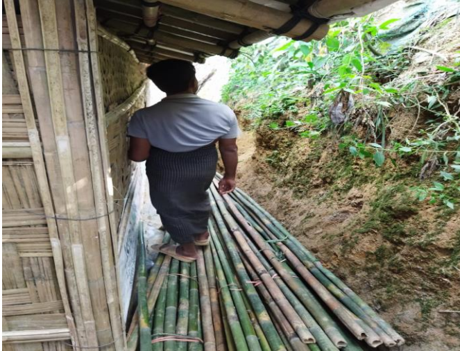
MTS construction under risk of land slide
