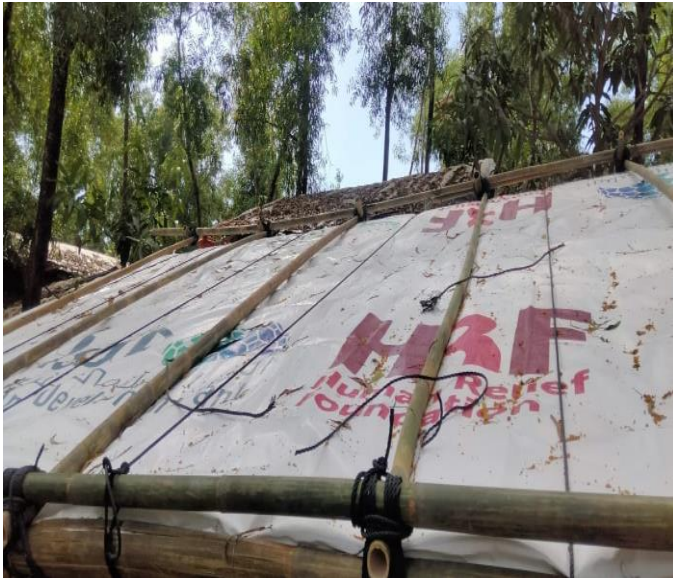
Wrongly set of branding tarpaulin
