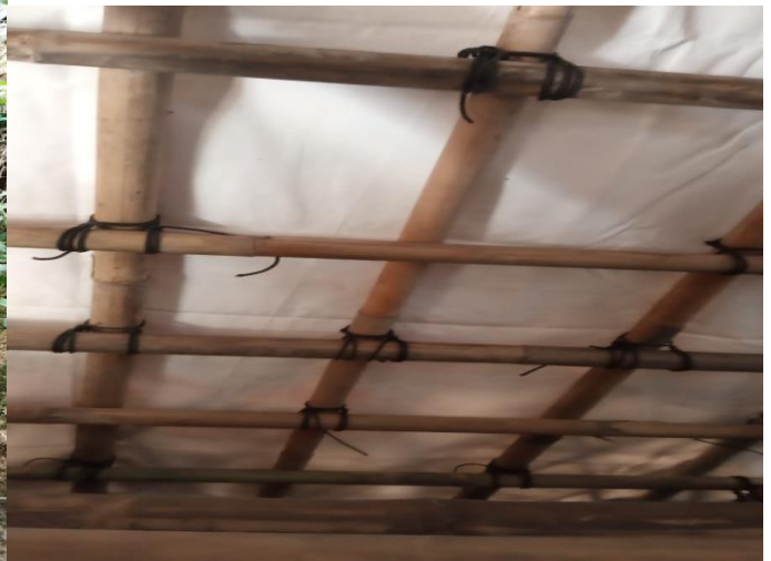
Not found tie of plastic rope
