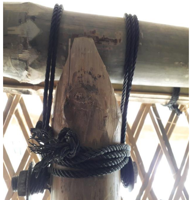
Rope tied is in wrong methodologically
