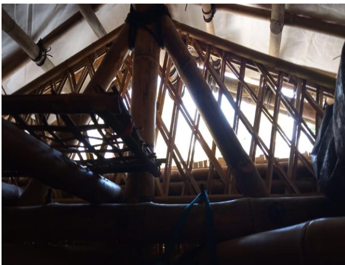
Granja's gap is too large
